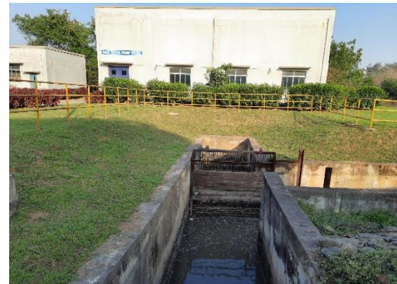
Automation of Rain water harvesting pumps
