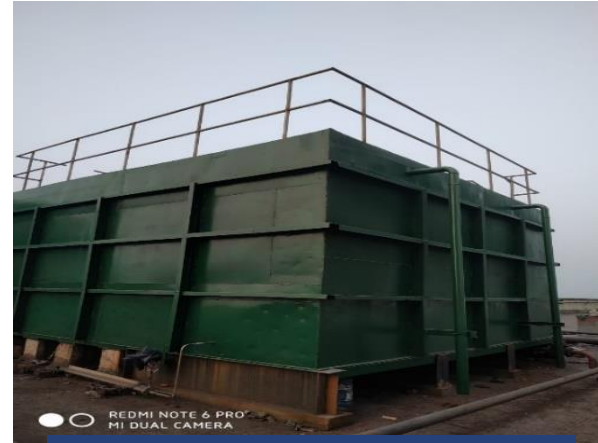
All Overhead tank level switch installation
